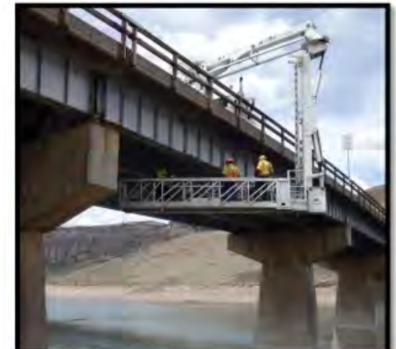
K-07-B, US 50 over Gunnison River/Blue Mesa Reservoir Identified as possibly being fabricated with T1 Steel
